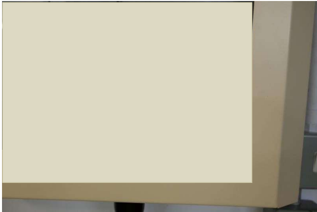
Fire alarm panel
