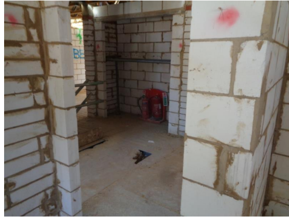
F Lane - typical interior, first floor, at this stage of construction - note fire point deployed
